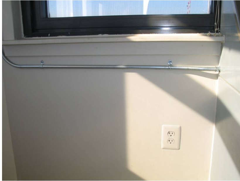
Figure 6 - Details Near a Large Window (South Tower)
